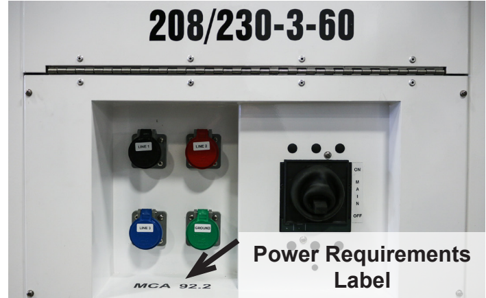
Figure 4 – Camlock Power Connections
